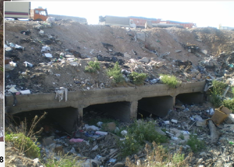
A branch of the river and seemed completely dry, which accumulate dirt, Sep 2007
